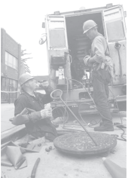
Employees of energy supplier ConEdison work on a street in the Astoria neighborhood in the Queens borough of New York, on 22 July, 2006. An estimated 100,000 residents of the borough entered the sixth day of a blackout as city officials said there was only a slight chance of restoring power before the end of the weekend. — INTERNET
