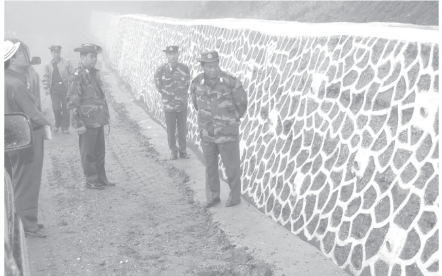
Lt-Gen Ye Myint of the Ministry of Defence inspects construction of retaining walls along Mindat-Matupi Road.—MNA
