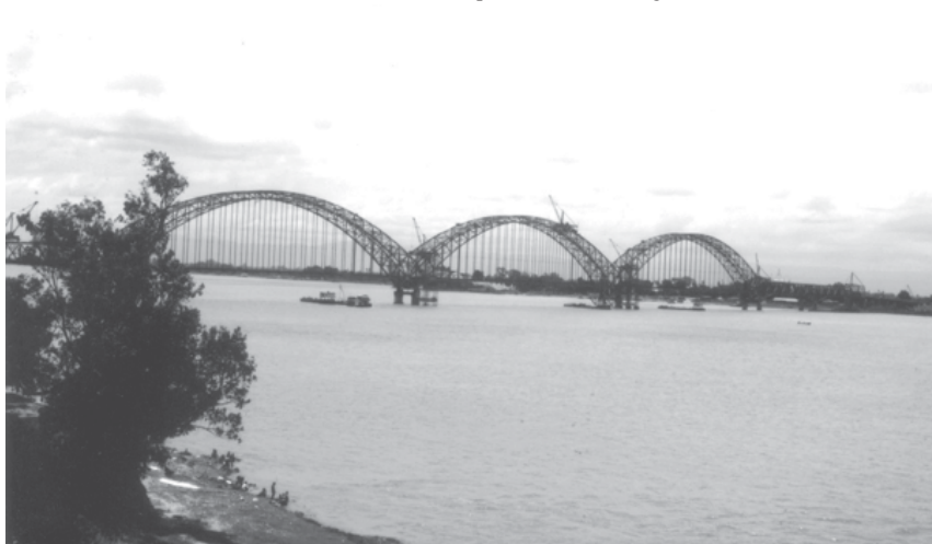
Progress of Ayeyawady Bridge (Yadanabon) construction project seen from Sagaing bank on 7-7-2006.
