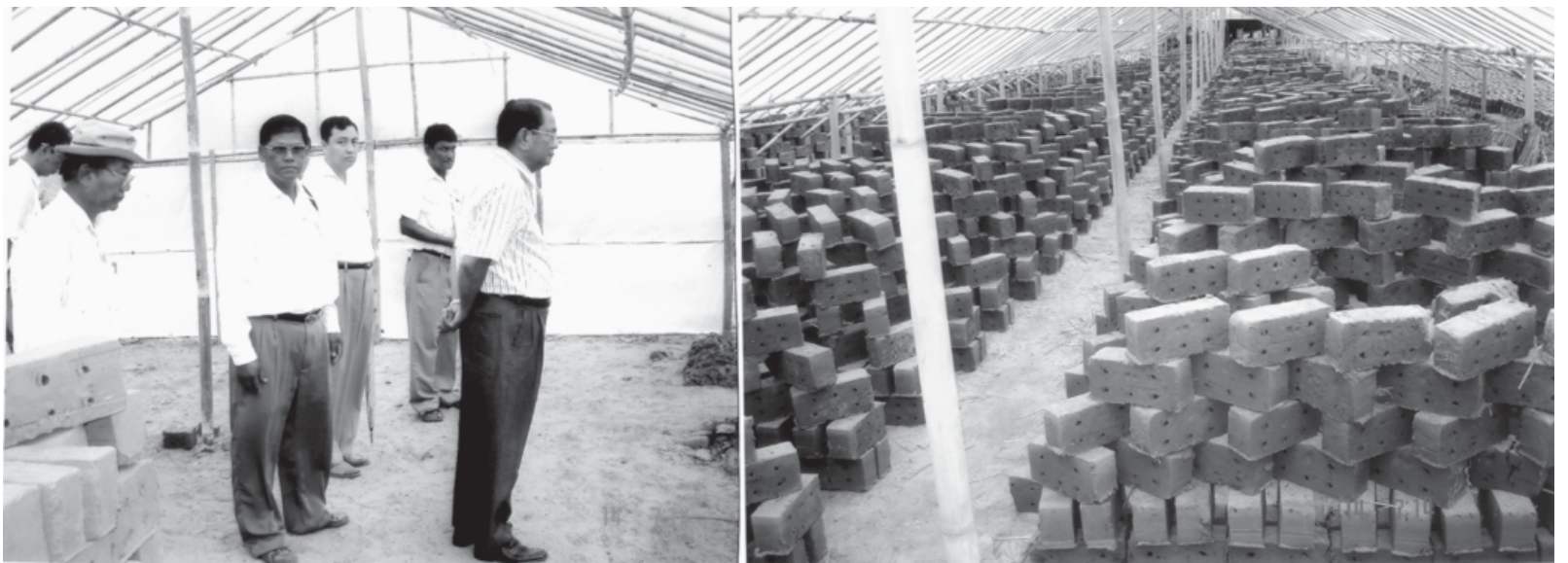
Minister U Aung Thaung inspects the drying of raw bricks at No 1 Brick Factory Project (Nay Pyi Taw).—INDUSTRY-1
