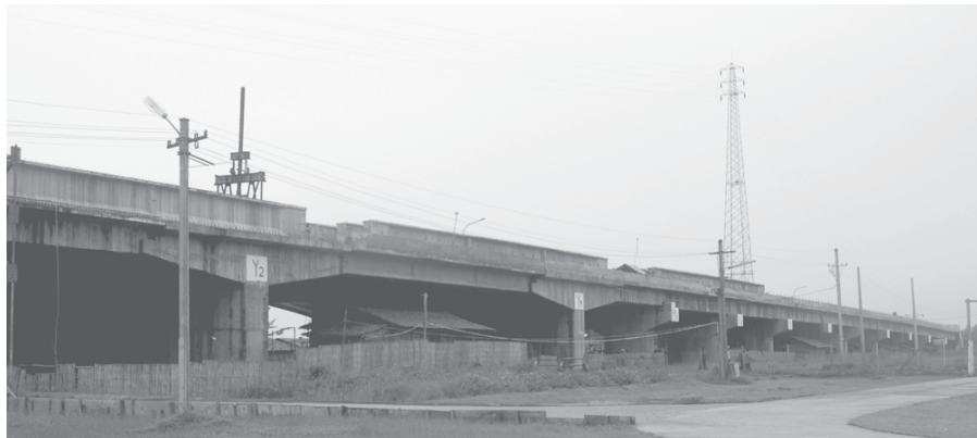
The photo shows progress of Yangon-Thanyin Bridge No 2 being built by Bridge Construction Special Group-1 of Public Works. — MNA
