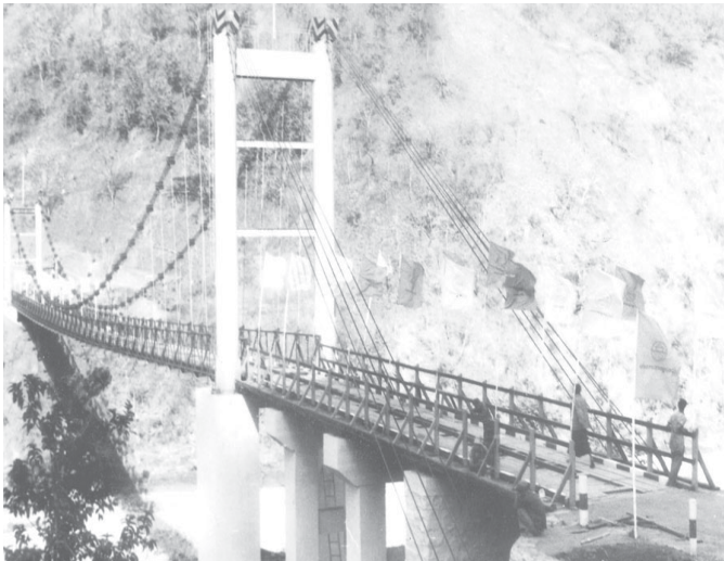
The 480 feet long and 10 feet and 9 inches wide Kattel suspension bridge across Manipur river is located in Tiddim Township, Chin State.
