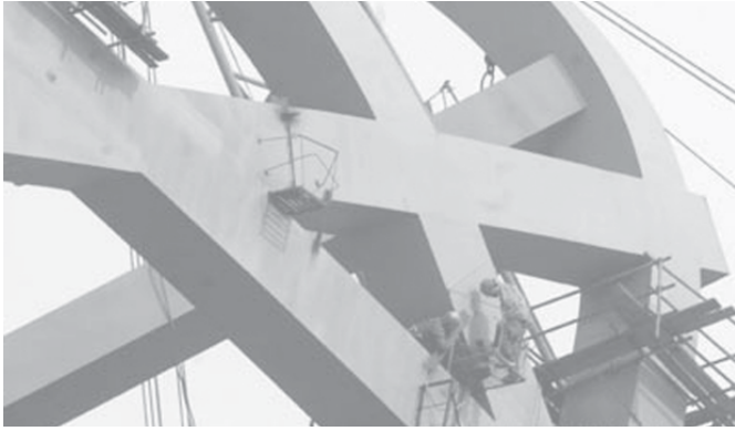
Builders work at the construction site of the Bird's Nest Stadium in Beijing, capital of China, on 5 July, 2006. The construction of the projects for the 29th Olympic Games are underway according to the plans by now. The construction of most stadiums and other related facilities including the athlete village are expected to be completed within this year.—INTERNET
