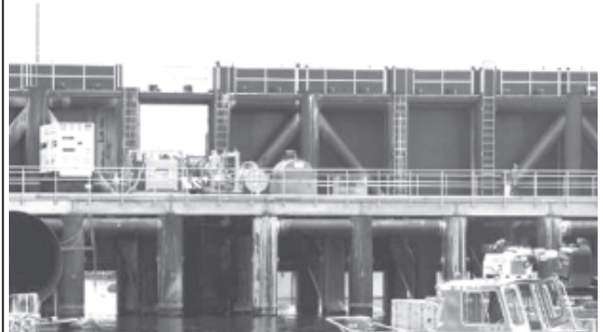
Construction crews work on the 17th street canal flood gates in New Orleans, Louisiana, on 1 July, 2006. The 17th street flood gates are designed to prevent water from Lake Pontchartrain from pushing into the canal during a storm. New Orleans residents fear inadequate repairs from Hurricane Katrina have opened the city to major flooding from less severe summer storms. —INTERNET
