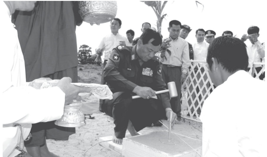
Commander Maj-Gen Khin Zaw drives a stake for construction of main building of Tele-Port in Yadanabon Myothit in PyinOoLwin Township. — COMMUNICATIONS
