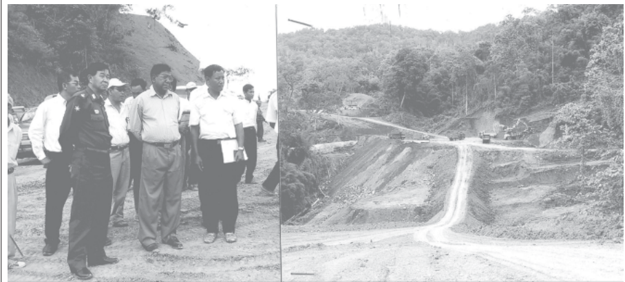
Minister Maj-Gen Aung Min inspects earth work for construction of railroad through Ponnya Mountain and laying of railroad in the tunnel. — RAIL TRANSPORTATION
