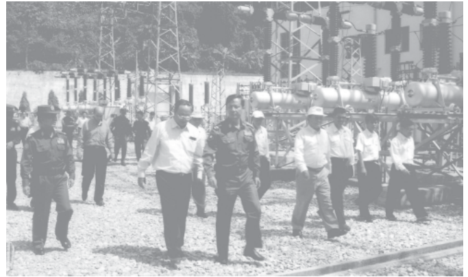
Commander Brig-Gen Thaung Aye and Minister Col Zaw Min inspect Biluchaung No 2 Power Plant. (News on Page 2)— ELECTRIC POWER NO 1
