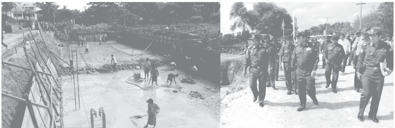
Lt-Gen Ye Myint inspects construction of a 500,000-gallon-capacity water tank and No 4 booster station in Aungmyethazan Township. — MNA
