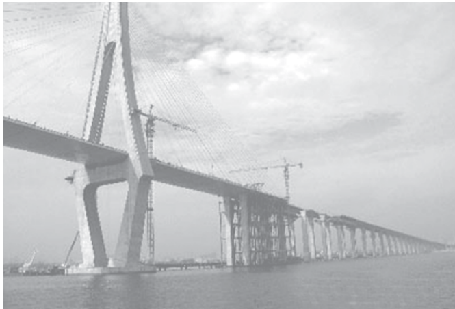
Photo taken on 21 June, 2006 shows the bridge under construction spanning Zhanjiang Gulf in Zhanjiang, south China's Guangdong Province. The two sections of the main bridge were joined on the morning of Wednesday. The length of the bridge is 3,981 metres and its main tower is 155.11 metres high.—INTERNET
