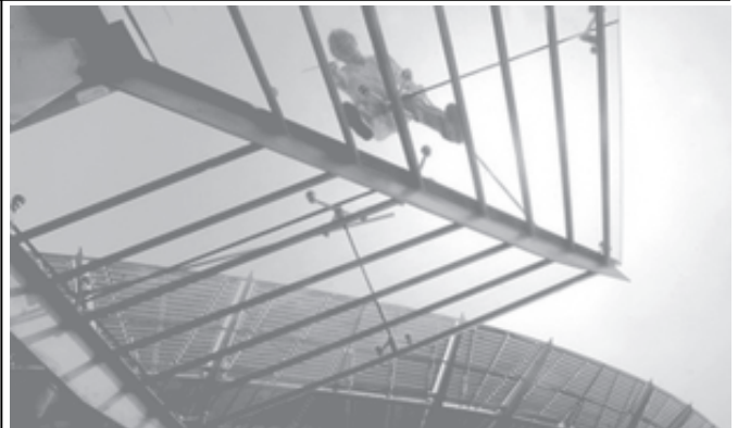
A worker cleans the roof of the disk-shaped Shanghai South Railway Station in Shanghai, in east China, on 19 June, 2006.— INTERNET
