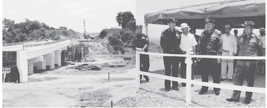
Lt-Gen Ye Myint of Ministry of Defence inspects construction of Mone Creek Bridge in Pwintbyu Township. — MNA
