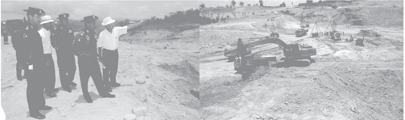
Lt-Gen Ye Myint inspects land preparations at Kyeoehn-Kyeewa Multi-purpose Dam Project in Pwintbyu Township. — MNA
