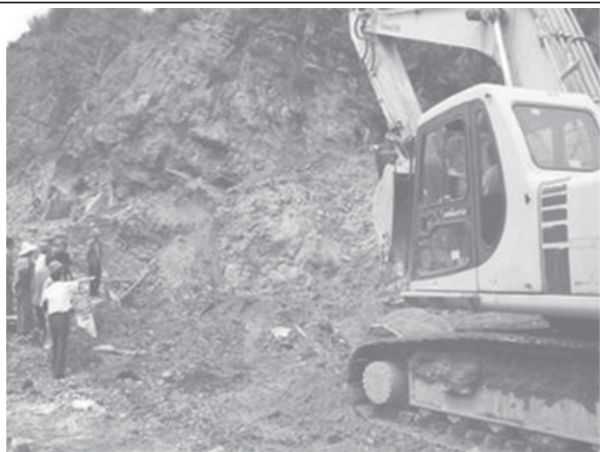
Rescue crew look for two missing workers at a construction site which collapsed in Xiuning County, east China's Anhui Province on 8 June, 2006.
