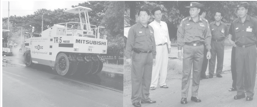
Mayor Brig-Gen Aung Thein Lin (C) supervises paving of Mindhamma Road. — YCDC
