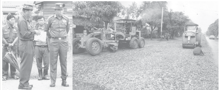
Mayor Brig-Gen Aung Thein Lin inspects preparations for upgrading of Thumingalar Street between Thitsar Street and Parami Road in South Okkalapa Township. — YCDC
