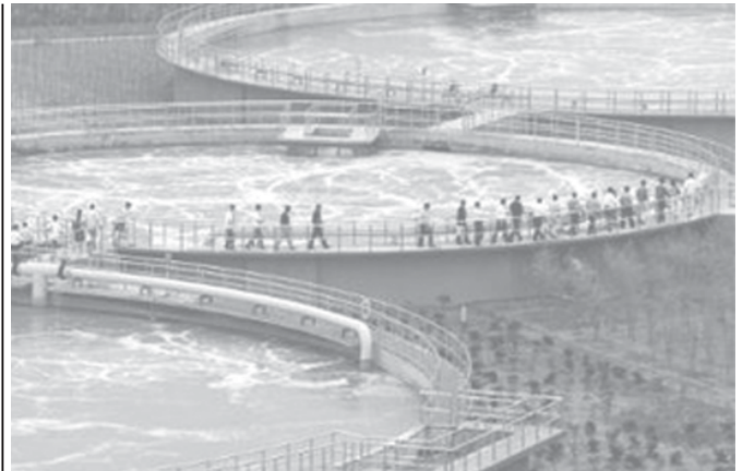
Visitors look at a sewage plant on the outskirts of Hangzhou, east China's Zhejiang Province on 5 June, 2006.—INTERNET
