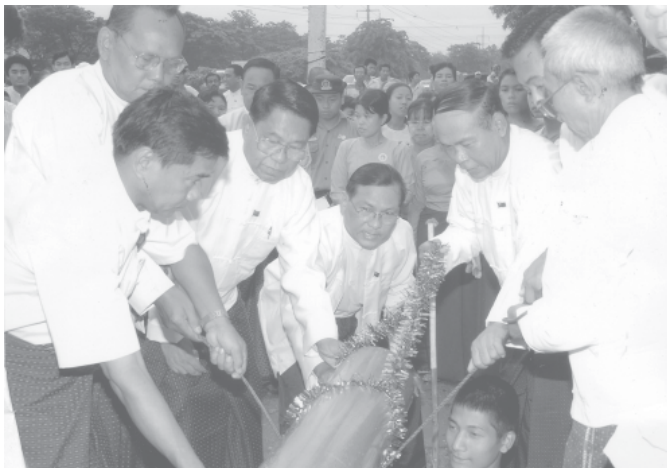
Mayor Brig-Gen Aung Thein Lin and Vice Mayor Col Maung Pa lay a pipe to supply water to Dawbon Township from Gyobyu reservoir.—YCDC
