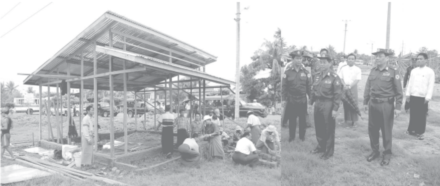
Lt-Gen Myint Swe of Ministry of Defence inspects construction of buildings at Shukhintha Tax-free Market. —MNA
