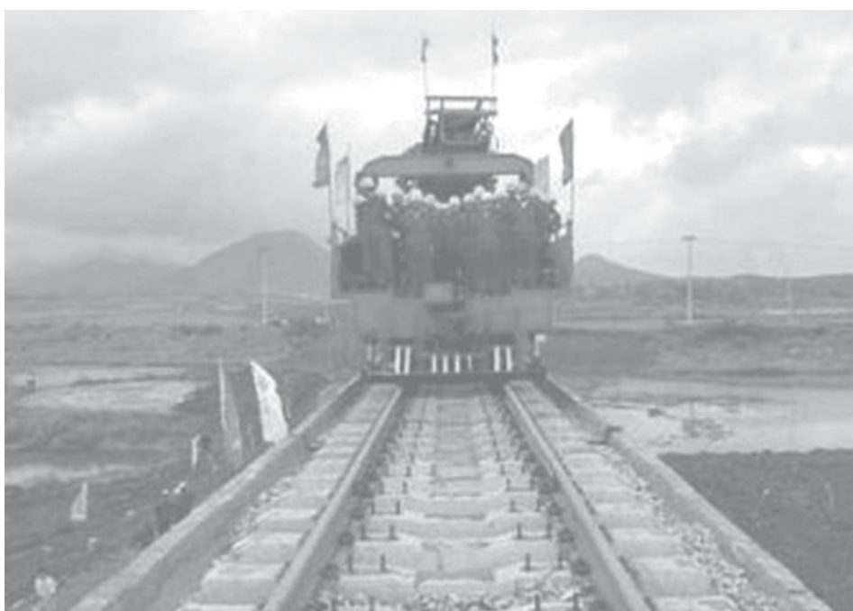
Labourers work at a construction site for a railway connecting Nanjing and Wuhan in Tongling, east China’s Anhui Province on 1 June, 2006.—INTERNET
