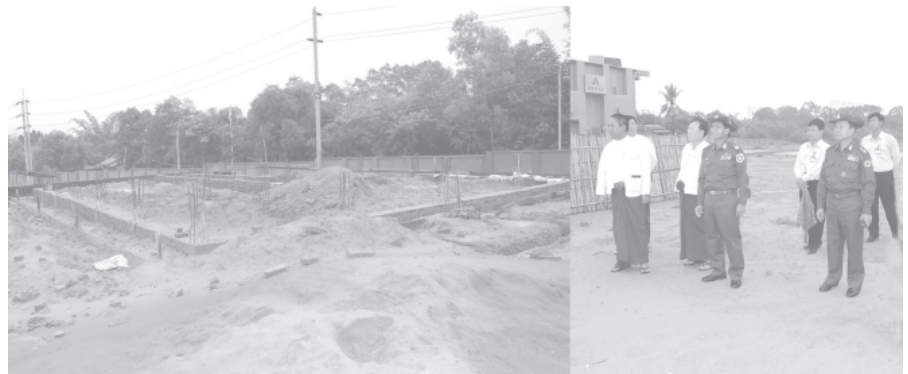
Minister for Electric Power No (2) Maj-Gen Khin Maung Myint at the construction site of 230 KV Sub-Power Station. — MNA
