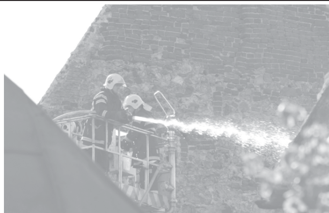
Firefighters spray water on the destroyed roof of a cathedral in Porvoo, Finland, on 29 May, 2006. The cathedral caught fire on Monday. The blaze had been extinguished, but the church roof was totally destroyed. The cathedral, one of the most famous ancient cathedrals in Finland, was the place where Tsar Alexander I opened the Diet of Porvoo in 1809. —INTERNET
