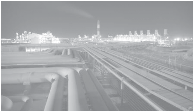
A general view of phases 2-3 of the South Pars gas field in Assaluyeh seaport at the Persian Gulf about 1400 km (870 miles) south of Teheran, Iran on 27 May, 2006. —INTERNET
