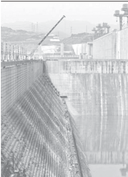
Workers install detonators to demolish the cofferdam of the Three Gorges Dam on the Yangtze River in central China’s Hubei Province on 29 May, 2006.—INTERNET
