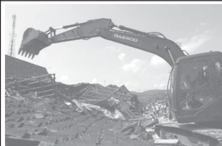
An excavator removes debris from the ruins of a house at the Imogiri District in Bantul, near Yogyakarta, on 28 May, 2006. Rescue workers dug desperately for survivors on Sunday and hospitals struggled to cope with the thousands of injured, a day after an earthquake killed more than 4,600 people on Indonesia's Java island. —INTERNET
