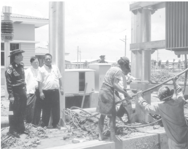
Minister Maj-Gen Khin Maung Myint inspects construction tasks of sub-power station in Hlinethaya. — MNA
