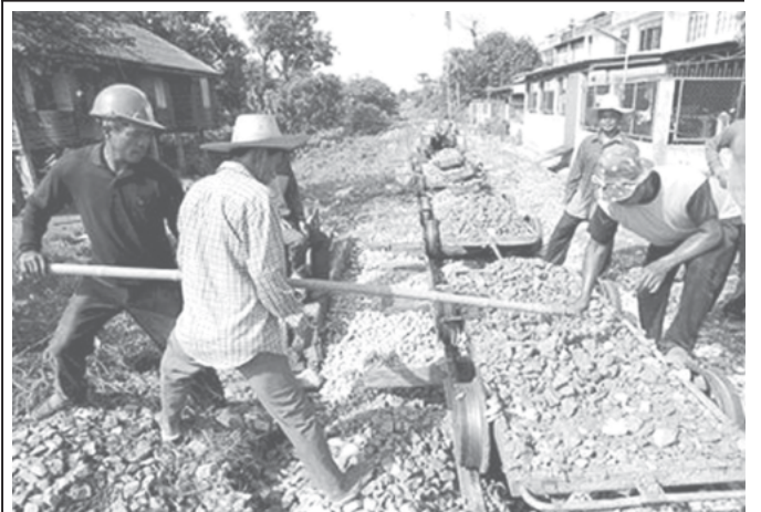
Thai workers repair a railway track after it was destroyed by floods in Sukhothai Province recently. The confirmed death toll in northern Thailand from floods and mudslides has risen to 62 while 53 people are still missing.—INTERNET
