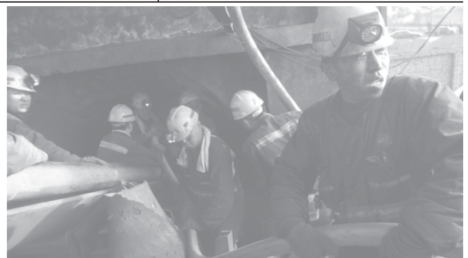
Rescuers equip a large diameter water pipe at the Xinjing Coal Mine in Zuoyun County, north China's Shanxi Province, on 23 May, 2006. By 6 pm on Tuesday, about 4,600 cubic metres has been pumped out of the mine, and water level in it began to fall. More pumps are to be used to speed up the pumping as 57 coal miners were still trapped by an underground flood since 18 May, 2006.—INTERNET
