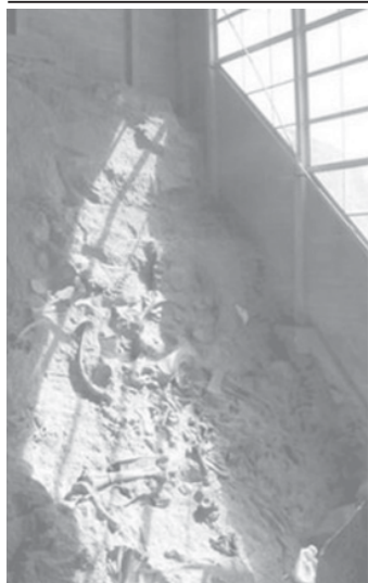
The visitor’s center encompasses a dinosaur bone yard embedded in sand on 18 May, 2006, at Dinosaur National Monument east of Vernal, Utah. The building, however, is shifting due to the unstable ground it was built on, resulting in cracked walls, uneven floors and jammed doors.—INTERNET
