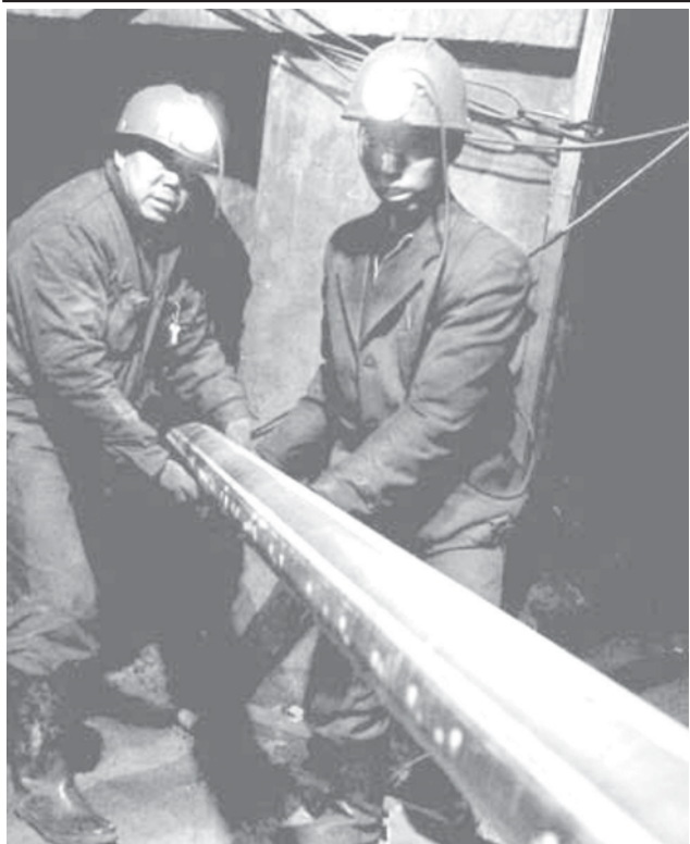
Rescuers install steel pipes to pump water out of the flooded shaft of a coal mine in order to rescue at least 44 still trapped underground in Zuoyun county, Shanxi Province on 20 May, 2006. A total of 145 miners were working underground when the flooding accident took place on Thursday night, and 101 managed to escape, rescuers said. —INTERNET
