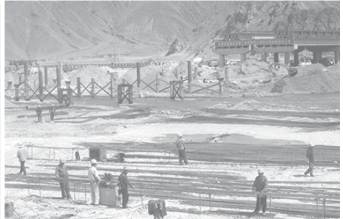
People work at the construction site of the Liuwu Bridge, a project for the Qinghai-Tibet Railway, in Lhasa, capital of southwest China's Tibet Autonomous Region on 11 May, 2006.—INTERNET
