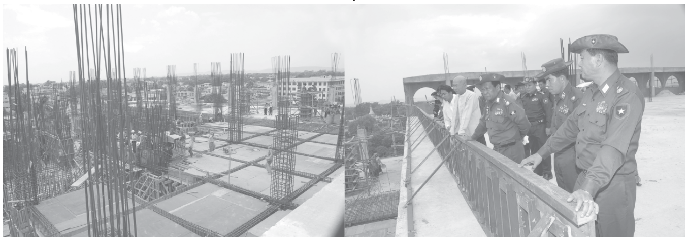
Lt-Gen Ye Myint inspects construction of six-storey Zaygyo Market building and 25-storey condominium tower in Mandalay. — MNA
