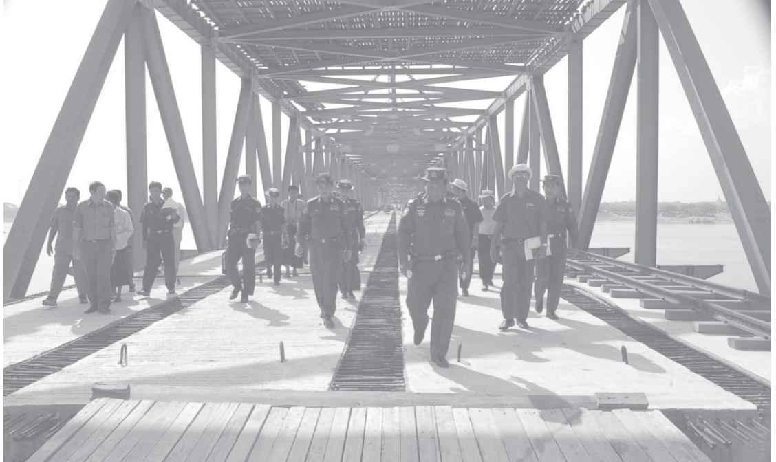
Lt-Gen Ye Myint (C) strolling on Ayeyawady Bridge (Yadanabon) during his inspection tour of the bridge under construction. — MNA
