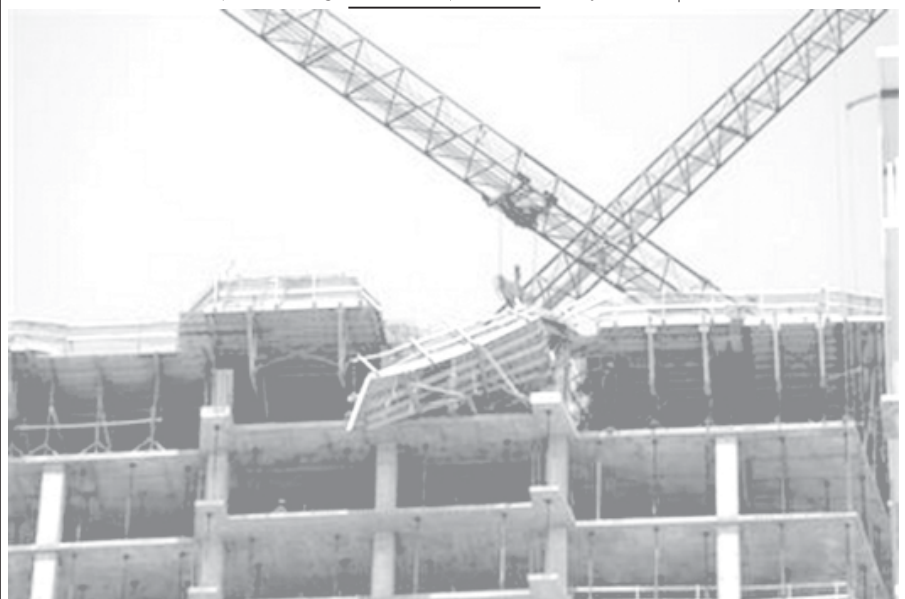
Three workers were killed when the wooden and metal frame seen in the centre of the photo, collapsed burying them under three feet of cement at a high rise hotel-condo project in Bal Harbour, Fla on 6 May, 2006.—INTERNET
