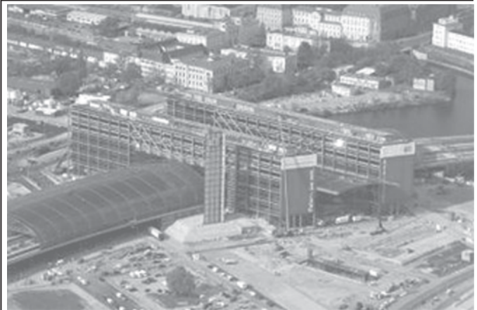
An aerial picture shows an unfinished new main central railway station in Berlin on 2 May, 2006. The railway station, Europe's largest, is scheduled to start operating at the end of May 2006, few weeks ahead of the start of the FIFA 2006 Soccer World Cup hosted by Germany. —INTERNET
