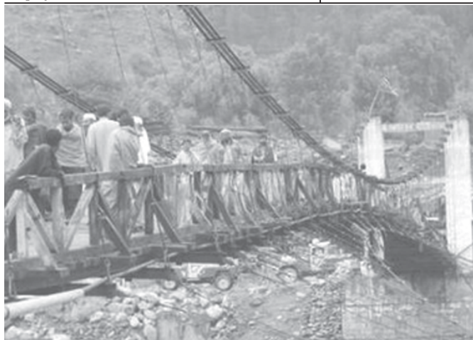
Pakistani earthquake survivors walk on a hanging bridge which was damaged in the quake in the earthquake-devastated town of Balakot, 180 km (112 miles) from Islamabad on 2 May, 2006. —INTERNET
