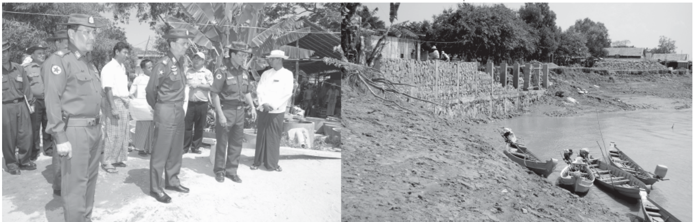
Secretary-1 Lt-Gen Thein Sein inspects bank erosion and construction of retaining walls at Htantabin circular road. — MNA
