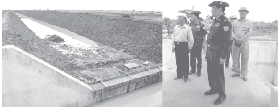
Commander Brig-Gen Hla Htay Win inspects Sitpin river water pumping project. — MNA
