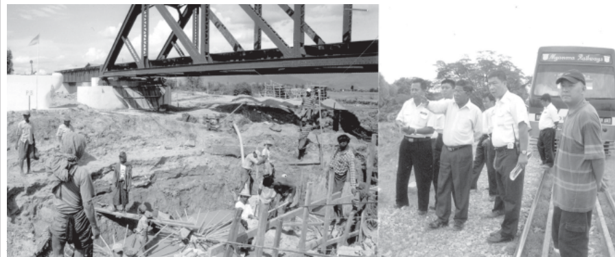
Deputy Minister U Pe Than inspects construction of a bridge on Yangon-Mandalay railroad. — MR
