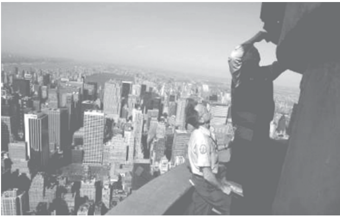
Workers replace a light fixture on the 103rd floor of the Empire State Building in New York on 11 April, 2006. As it turns 75 years old, the iconic building has fallen on hard times. But its supporters say it is also poised for a comeback. —INTERNET
