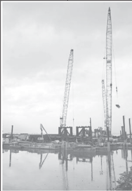
Cranes are used to construct a floodgate between the Seventeenth Street Canal and Lake Pontchartrain in the Lakeview area of New Orleans on 26 April, 2006. INTERNET
