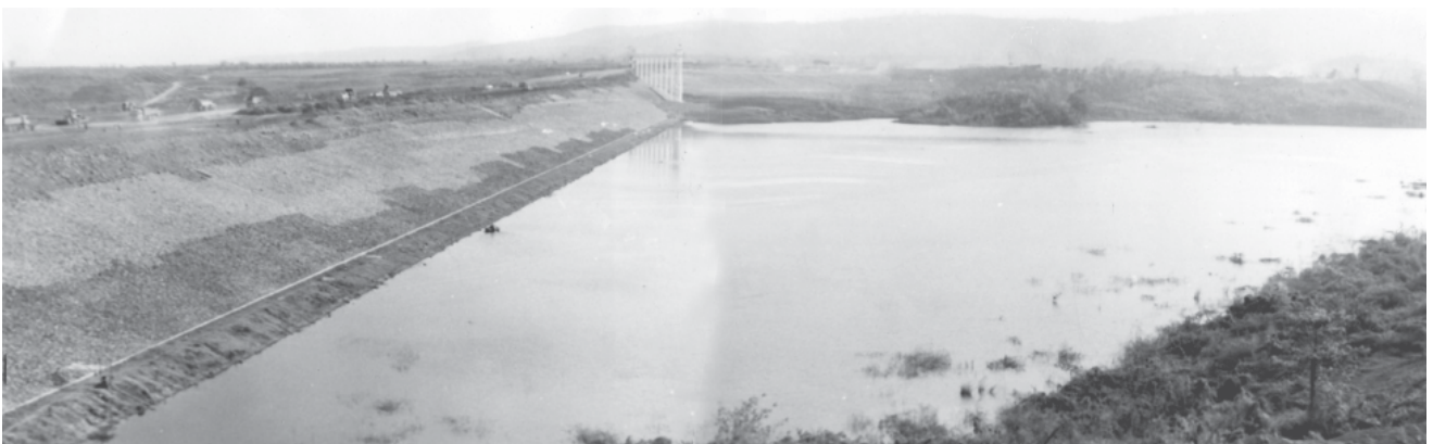
Ma Mya Dam is being built by damming Ma Mya Creek near Hmyinwataung Village in Myanaung Township, Ayeyawady Division.
