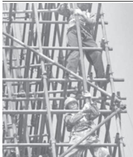
Chinese men work on the scaffoldings at a construction site in Nanjing, the capital of east China's Jiangsu Province, on 20 April, 2006.
