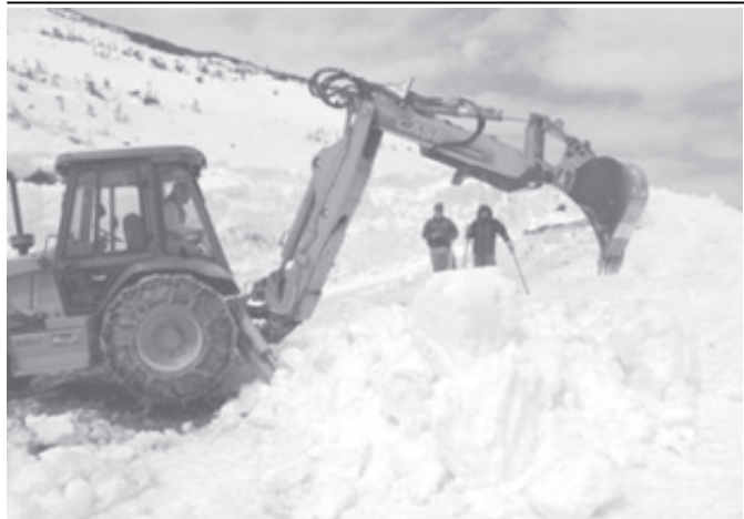
Road crew members for the Mount Washington Auto Road work on removing snow on 19 April, 2006 from the highest peak in the northeastern United States. They hope the road will be open by the end of April.—INTERNET
