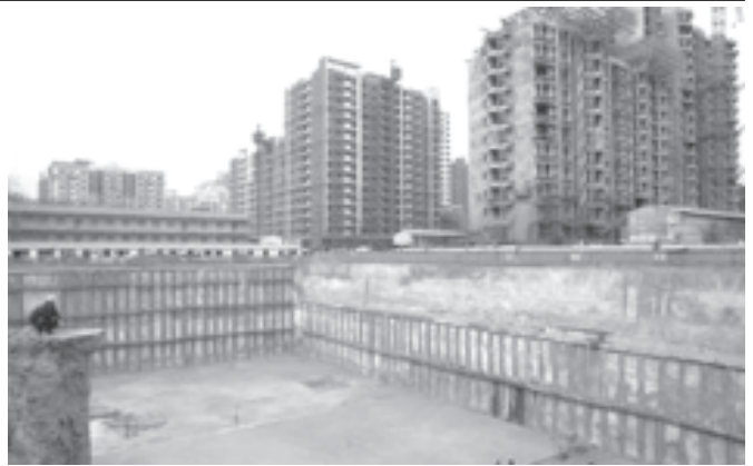
A Chinese worker perched precariously over a gigantic hole construction as the foundation of another building project in Beijing, China on 17 April, 2006. President Hu Jintao announced Sunday that the economy grew 10.2 percent in the first quarter — more than 2 percentage points above the official target. — INTERNET
