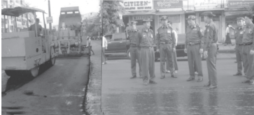
Commander Brig-Gen Hla Htay Win and Mayor Brig-Gen Aung Thein Lin inspect the laying of asphalt on West Race Course Road in Tamway Township. — MNA
