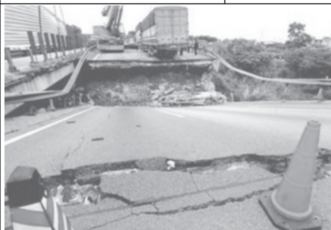
A collapsed section of the Shenzhen and Shantou expressway is seen in Shenzhen, Guangdong Province, China, on 16 April, 2006.—INTERNET
