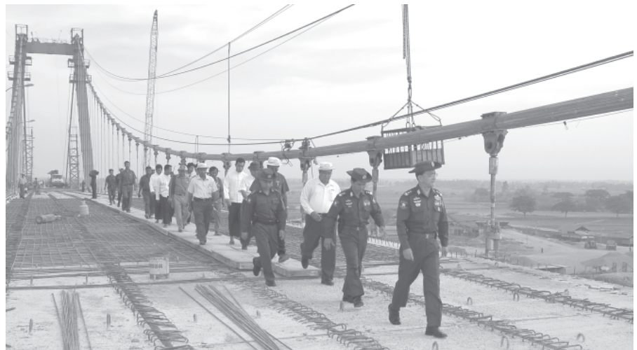
Secretary-1 Lt-Gen Thein Sein inspects progress in construction of Twantay Bridge. — MNA
