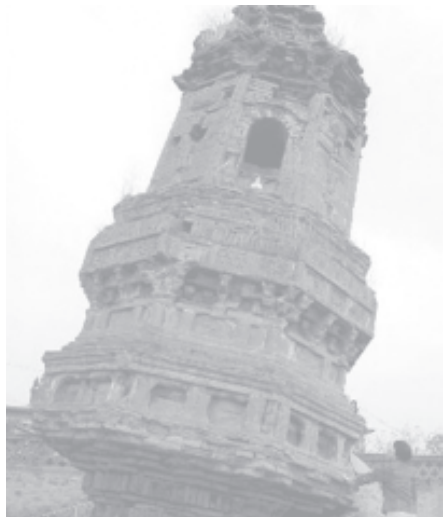
Built in Liao Dynasty, the leaning tower in Huludao, northeast China's Liaonin Province is now 10 metres high and inclines 12 degrees to the northeast. —INTERNET
