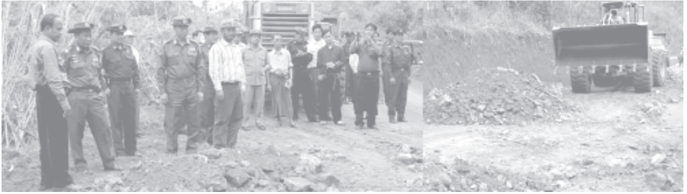
Lt-Gen Ye Myint of the Ministry of Defence oversees progress in paving gravel road with the use of heavy machinery at mile post No 34/35 in Myitkyina. (News on page 1)—MNA
