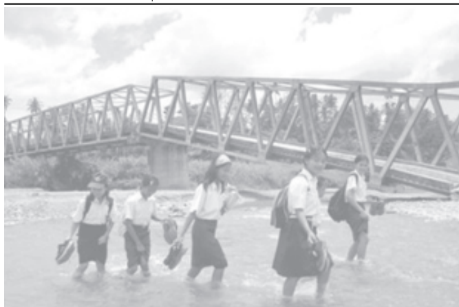
Students walk across a shallow river as a bridge damaged by March 2005's earthquake is seen on the background, in Idano Gawo, Nias island, Indonesia, on 3 April, 2006. —INTERNET
