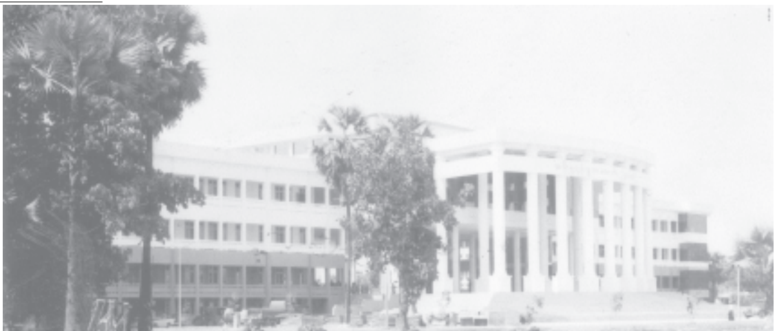
Lt-Gen Maung Bo of Ministry of Defence inspects progress in construction of Government Computer College in Hpa-an. —MNA
