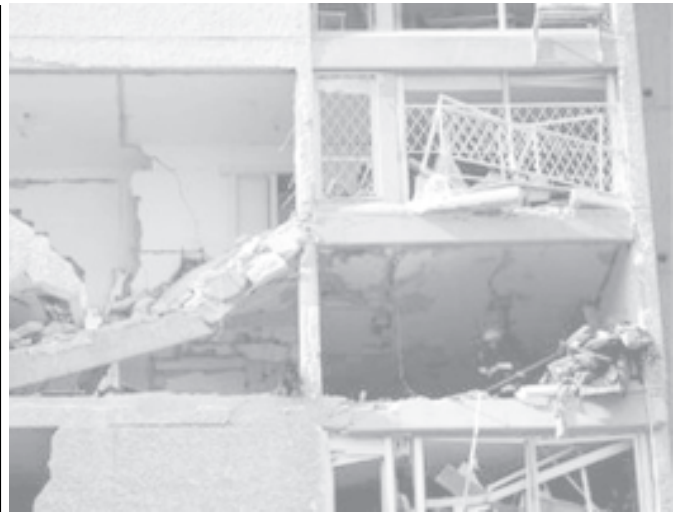
A fire-fighter stands in an apartment building after an explosion in Haifa, Israel, on 30 March, 2006. An explosion, apparently caused by a gas canister, ripped through the apartment building on Thursday, injuring seven people, Israeli radio stations reported. —INTERNET
