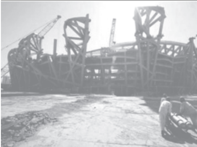
Chinese men work at the construction site for the Olympic stadium in Beijing, on 28 March, 2006. —INTERNET
