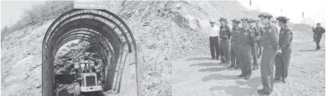
Prime Minister General Soe Win inspects construction of underground diversion tunnel at Myogyi Multi-purpose Dam Project in Ywangan Township. — MNA
