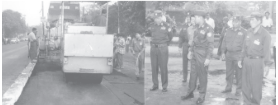
Mayor Brig-Gen Aung Thein Lin inspects laying of asphalt on U Chit Maung Road in Bahan Township. —MNA
