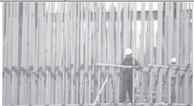
Chinese workers work in a construction site in downtown Shanghai on 20 March, 2006. China must press ahead with reforms to help sustain strong economic growth that has fuelled foreign pressure on its trade and currency policies, a top government think tank said in a report published on Monday.—INTERNET
